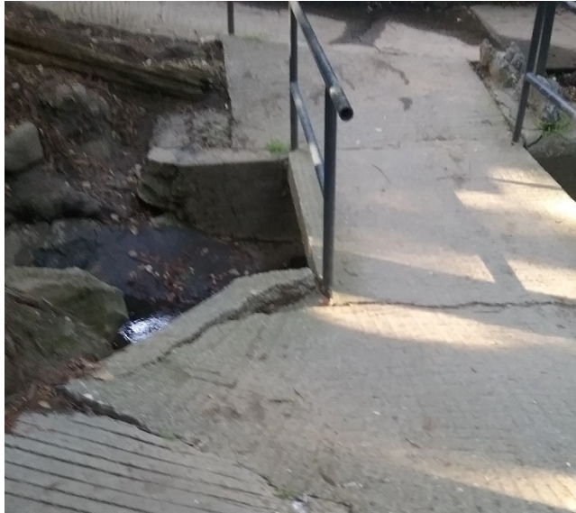
View of concrete bridge in Piedmont Park to be replaced (Project 36M)
